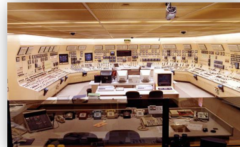
Nuclear Power Plant Simulator
